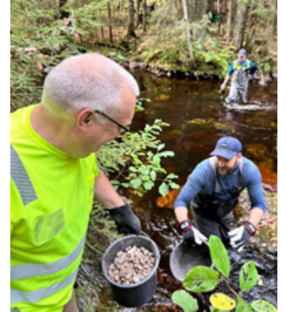
Enhancing the habitat conditions for the endangered brown lake trout in connection with the Niinimäki wind farm.
