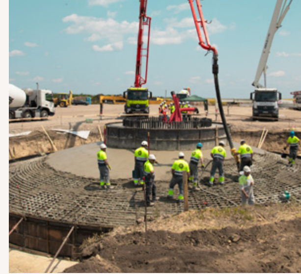
Green Breeze wind farm is OX2’s first project to be constructed in Romania.
