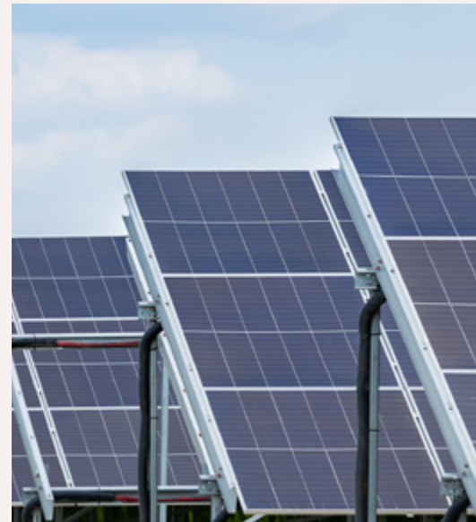
Rutki Solar Farm in Poland, our first fully owned project as an independent power producer, began delivering electricity to the grid in July 2025.
